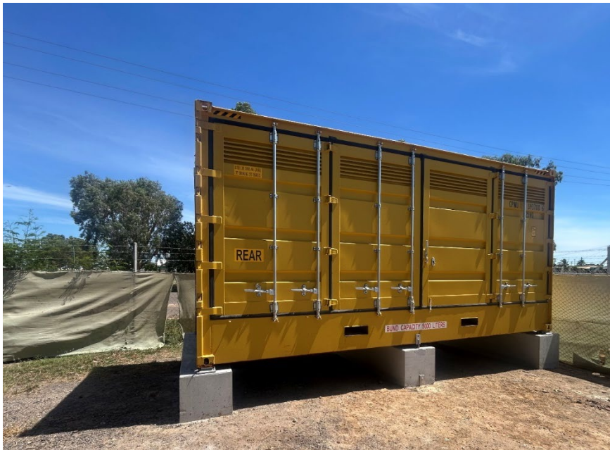
Figure 4: The chemical container installed.
