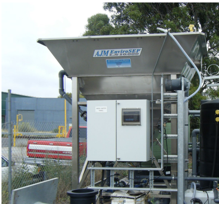
Figure 1: Lamella clarifier located at Richmond
