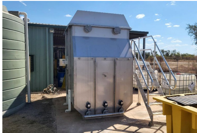
Figure 1: The new Clarifier at Gregory Water Treatment Plant
